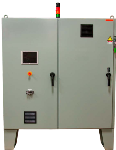
This panel is a Bio Genset control designed by an ECT customer. ECT procured the material, fabricated the panel and performed point to point inspection prior to shipment.
