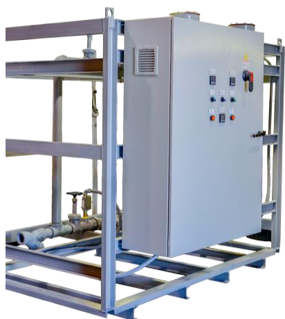
This panel is for a process heating application. ECT designed, fabricated, installed and wired the control panel on the customer's process equipment.
